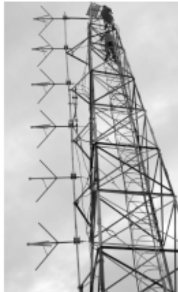
Fig 10. Circular Antenna System
